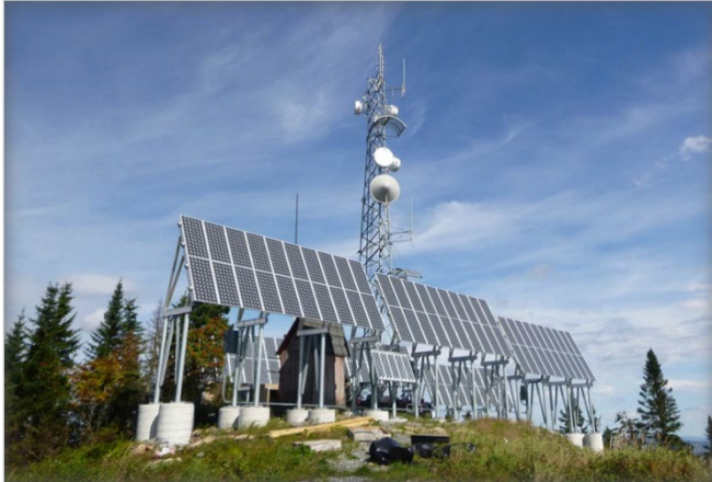
Figure 4: RF Site with Solar Power Plant
