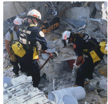
Search and rescue operation following gas mainline explosion. Courtesy of FEMA.
