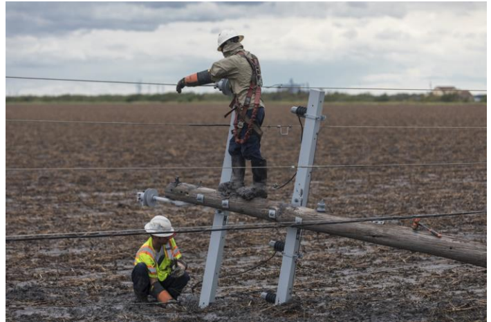
Power utility personnel repair electrical transmission lines outside the town of Rockport, TX in response to Hurricane Harvey, 2017 (Source: FEMA)
