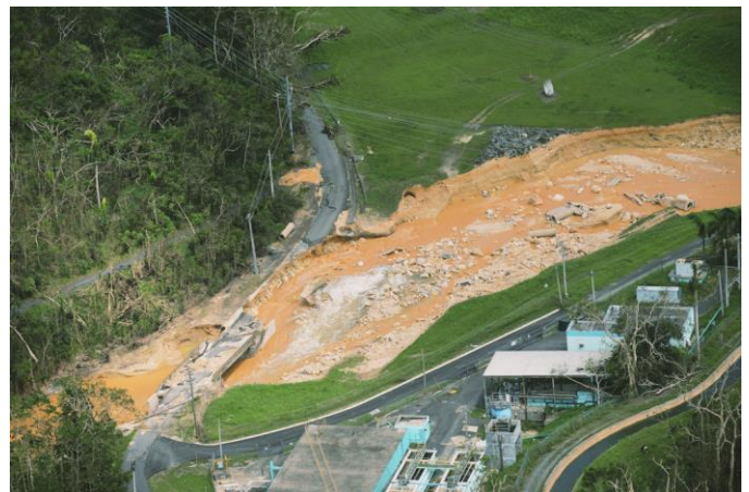
Guajataca Dam damage in Quebradillas Municipality caused by heavy rains from Hurricane Maria, 2017 (Source: FEMA)
