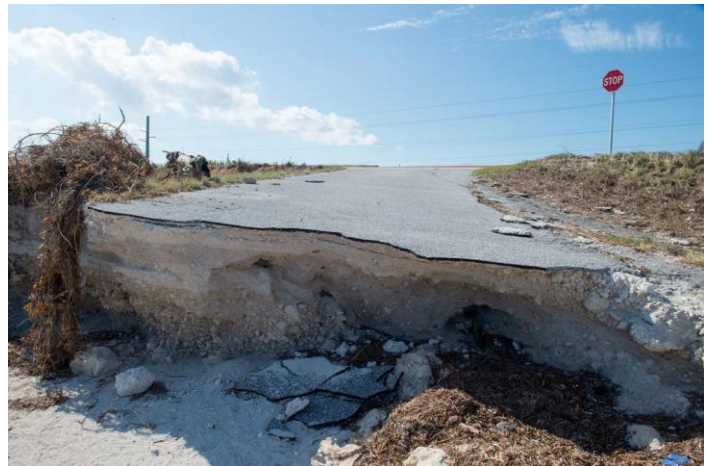
Campground road off of Overseas Highway collapsed after Hurricane Irma in Big Pine Key, Florida on Sunday, September 17, 2017 (Source: FEMA)
