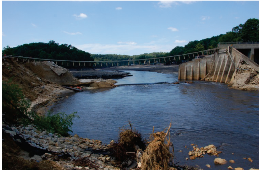
Following heavy rains in 2010, a torrent of water from a breach in the Lake Delhi Dam in Iowa left little in its wake and damaged homes and businesses downstream. (Source: FEMA, Josh deBerge)
